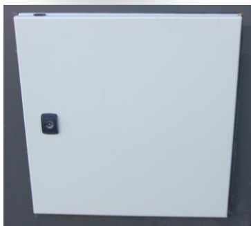
External view on electric box.
