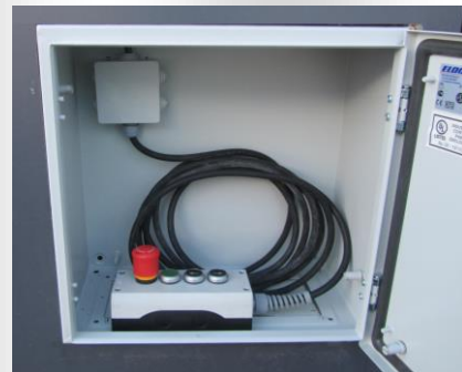
Internal view of electric box with wire control unit and different length of electric cable.
