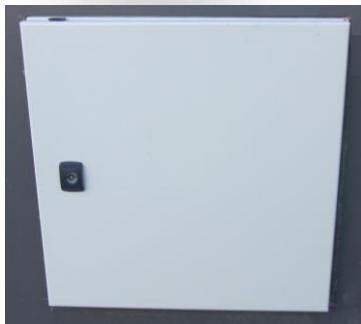
External view on electric box.
