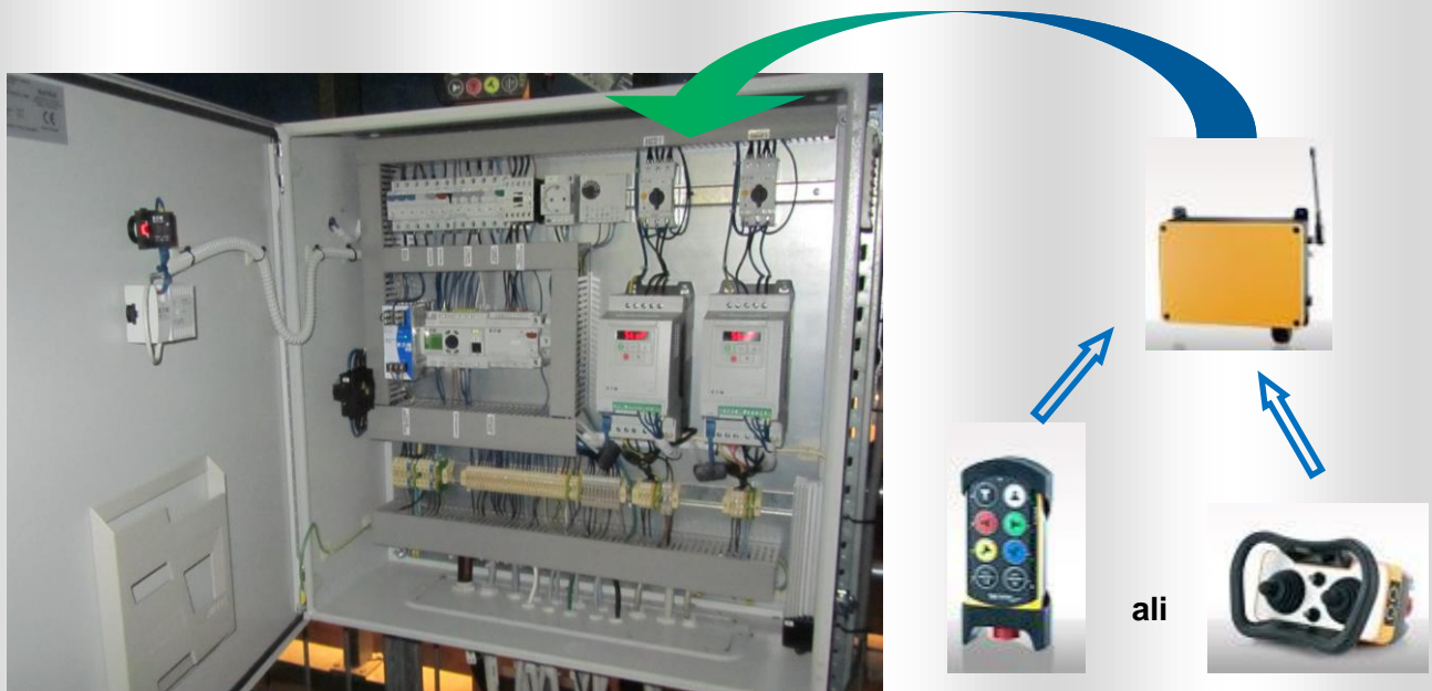
The internal appearance of the electrical box and remote control, FALUN 2013.
