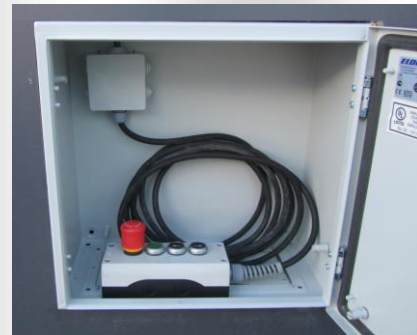
Internal view of electric box with wire control unit and different length of electric cable.
